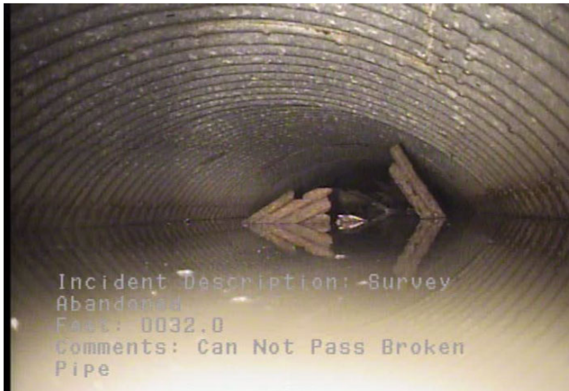
Sides failing, bottom of pipe sticking up- causing more than ½ pipe blockage.
