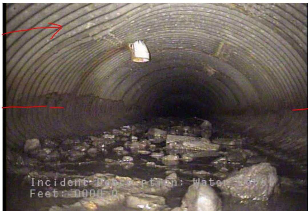
Sides failing- top starting to buckle due to deterioration.
